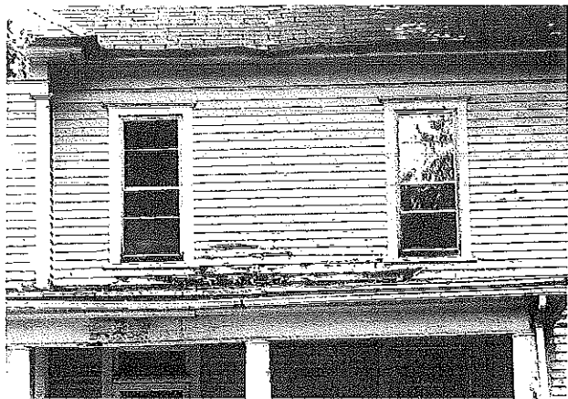
These replacement metal windows are inappropriate. A two-over-two pattern with horizontal muntins is not historically authentic, and neither is the metal material.
