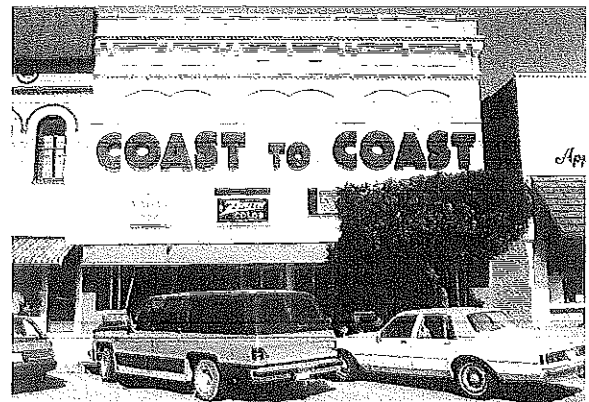
The second floor openings of this building have been inappropriately infilled with brick and an over-sized sign has been applied over this area. What was once a fine building with interesting brick detailing has suffered an almost complete loss of historic integrity.
