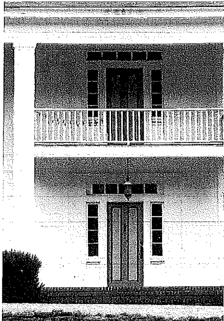
The transoms and sidelights of the Phillips-Smith House in Hogansville are important architectural details, helping to define the character of this particular house.
